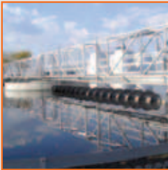
WASTE WATER RECLAMATION
