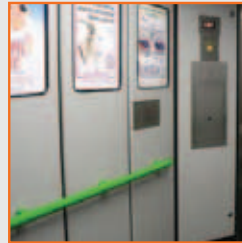
LIFT MONITORING SYSTEM
