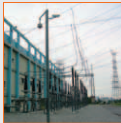
POWER TRANSMISSION MONITORING
