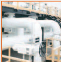
LIQUID AND GAS PIPELINES AND FLOW COMPUTER MONITORING
