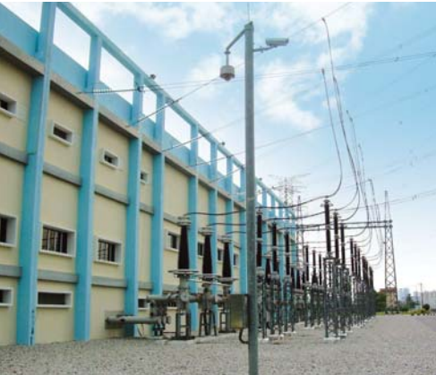
Power Transmission Monitoring
