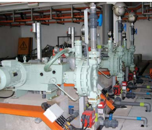
Process Control and Plant Monitoring
